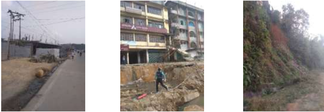
Picture 8: Sewerage Lines in ICR
