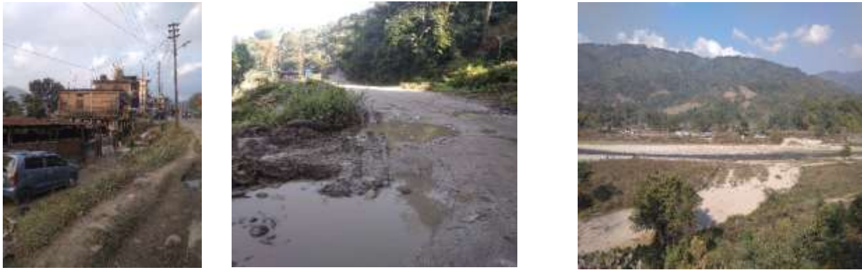
Picture 9: Storm water Drain Condition in ICR
