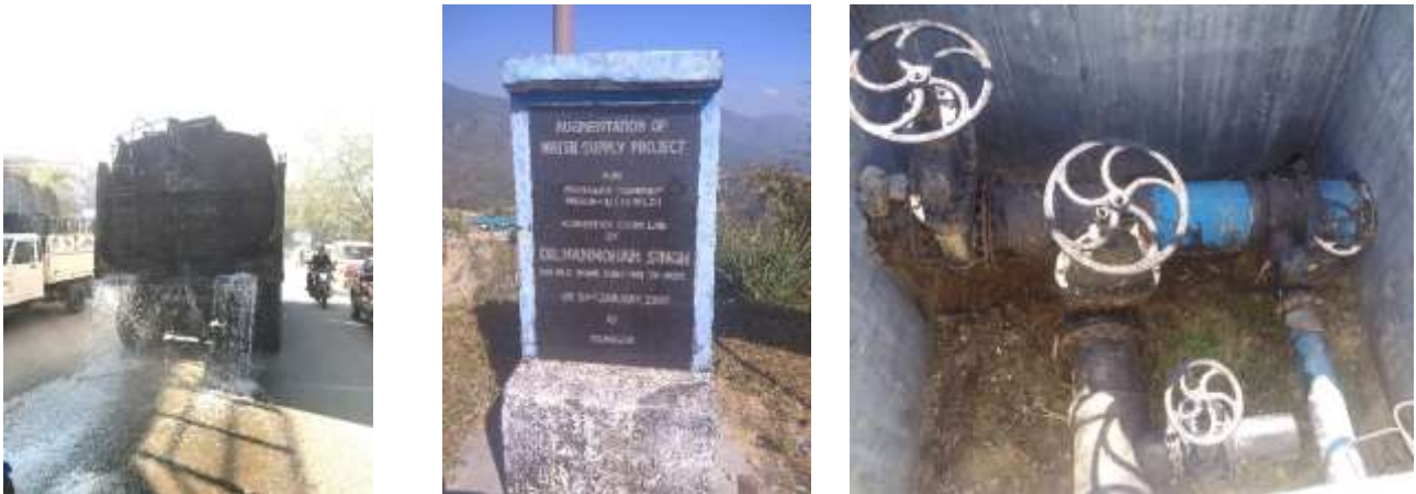
Picture 7: Water Supply in ICR
